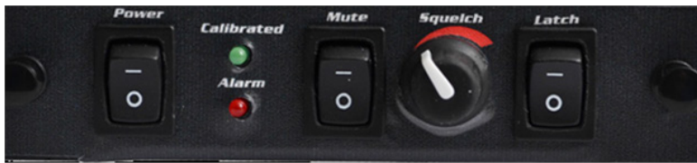
Fig C: Zone Control Unit front panel
